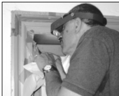
Paint and finish expert Matthew Mosca carefully removes layers of paint to reveal original finishes.
