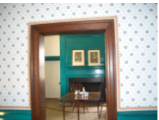
Views of the process of restoration of the Main Hallway: Replastering follows re-wiring; paint samples provided by Matthew Mosca are used as a reference; the painting of 4 layers of verdigris over paint is completed, and the wallpaper is installed.
