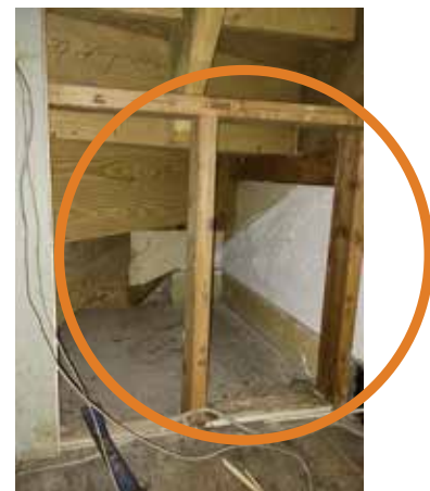
This photo is more interesting than it seems. It's the space that was the closet under the stairs in the corner of the farm office. The plastered wall on the right shows the original slope of the original stairs that were in this position in the Croghans' day, which were less steep than the current stairs built by the restorers in the 1960s. So, the stairs on the second floor opened closer to the hallway, and the cutout in the floor probably once allowed for the right closet door in the bedroom to actually open all the way -- one of the puzzles of the room's layout.
