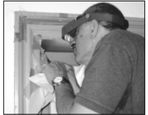
Paint and finish expert Matthew Mosca carefully removes layers of paint to reveal original finishes.
